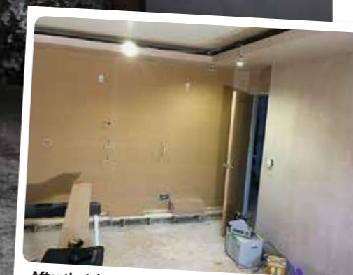
After the initial planning stage, the installer's first task was to strip out the existing kitchen and prepare the room for its home cinema transformation
